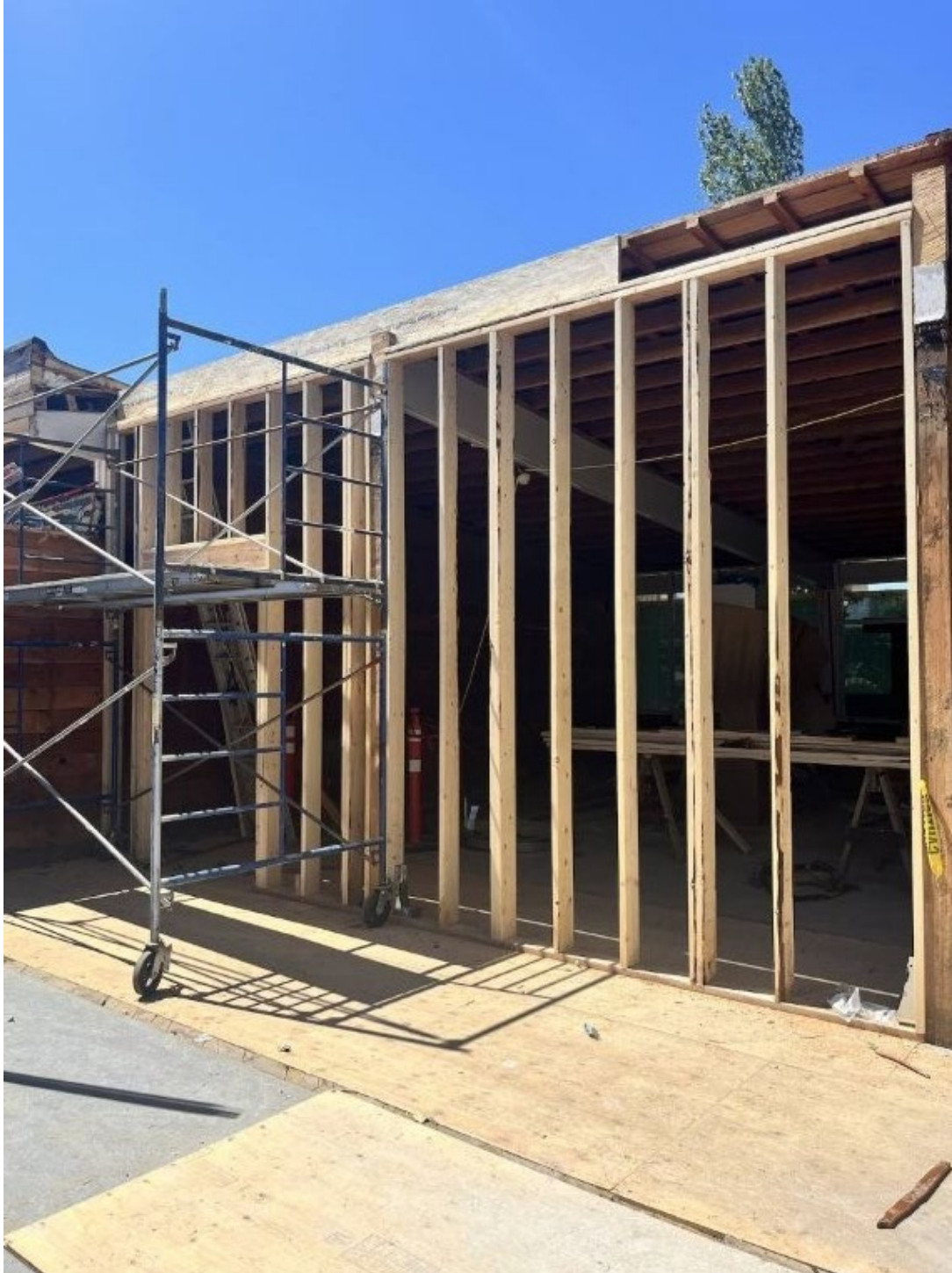
Classroom Seismic Framing
