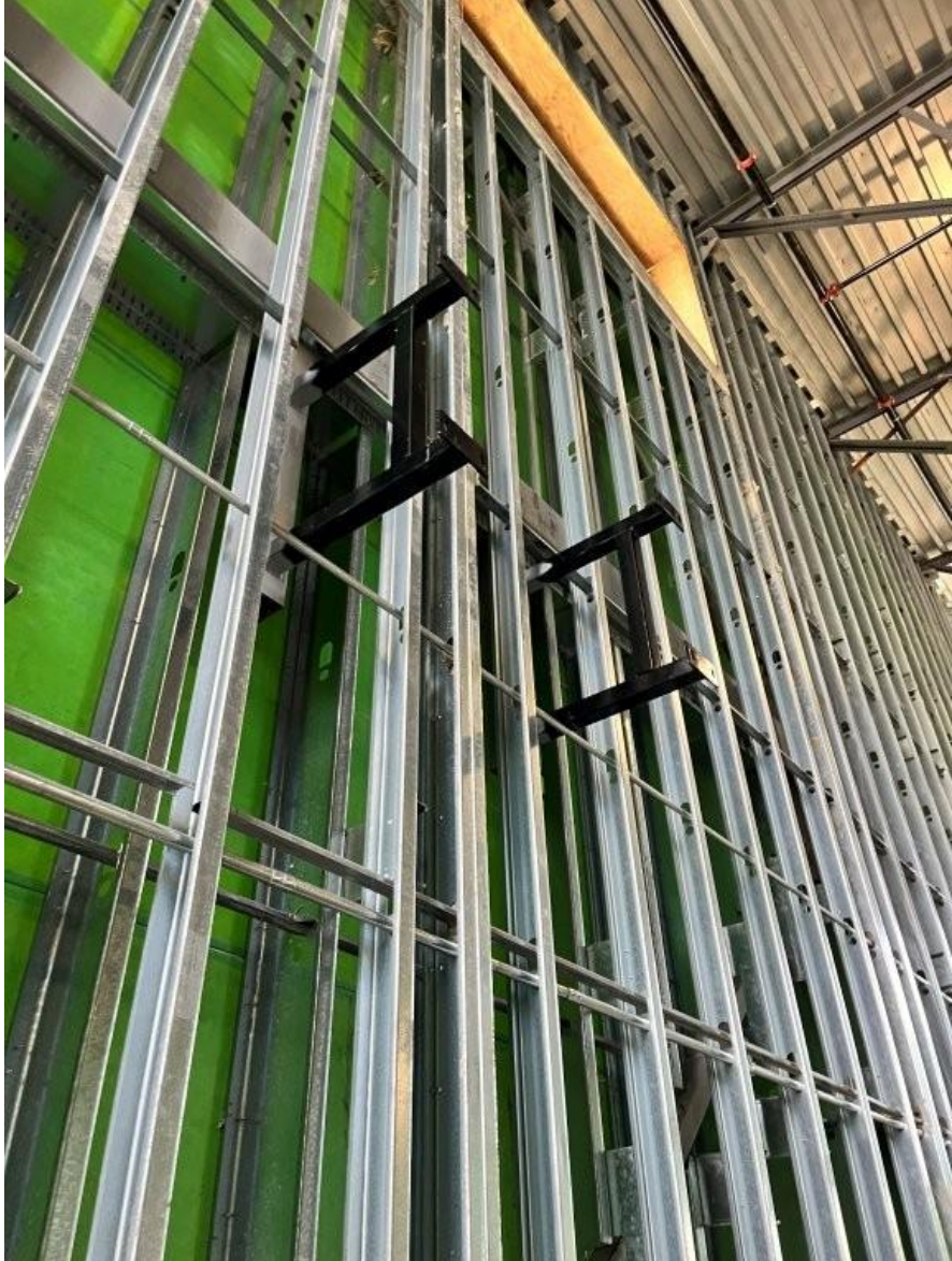
New Gym – Basketball Supports
