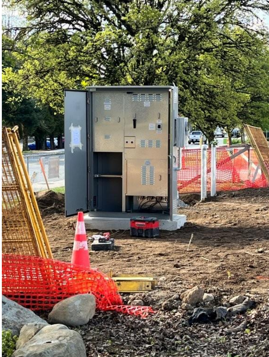
New BC Hydro Metering Kiosk
